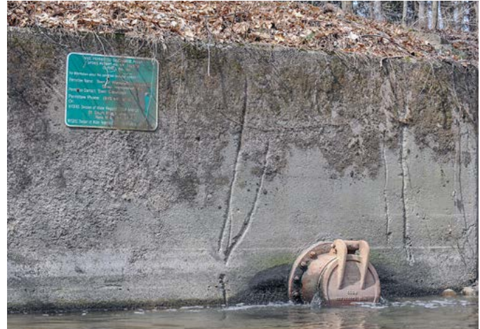
SPDES outfall site. © E. Vail
