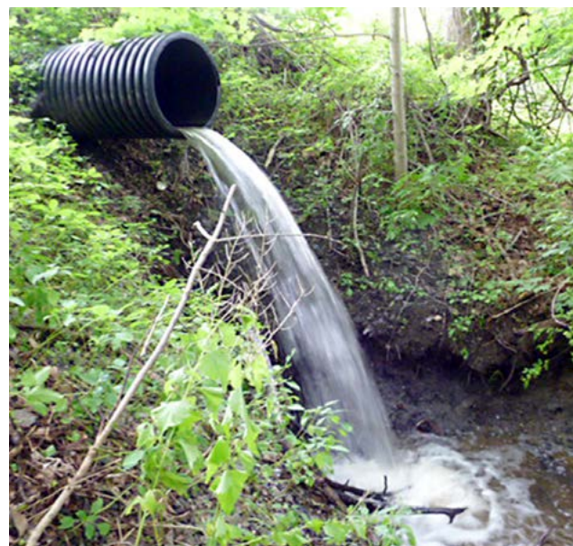
Hanging culverts prevent fish from travelling upstream. © M. Adamovic
